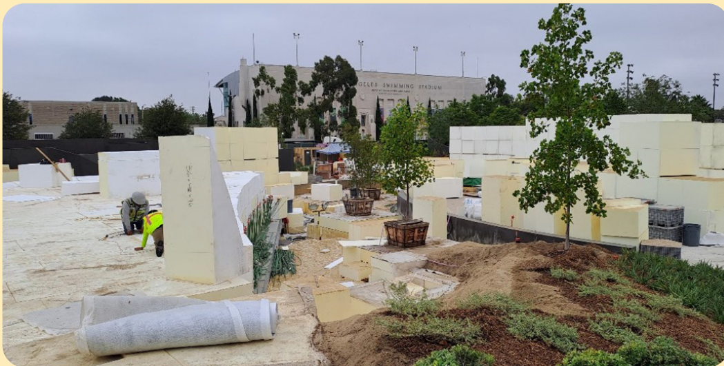
Figure 8 Foam blocks being used as an alternate light weight sub surface fill material instead of traditional quarried materials
