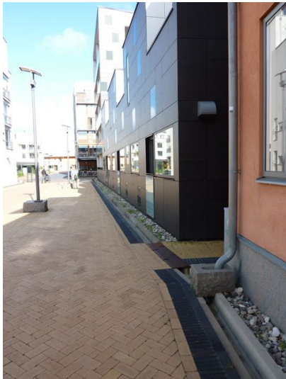
Figure 11 - downpipes feed directly into open drains
