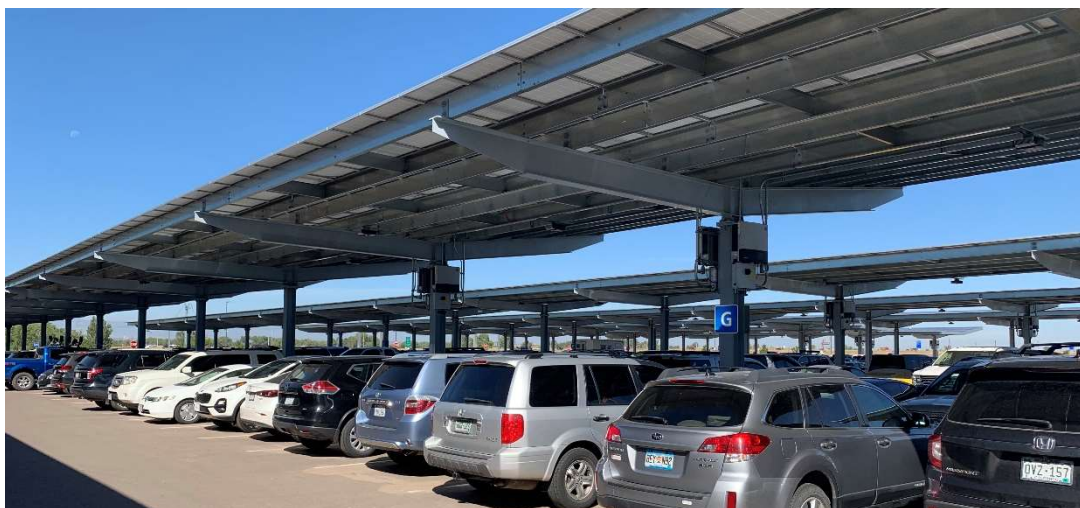
Figure 52 – The vehicle shelters at Panasonic City NOW – consisting of PV Panels
