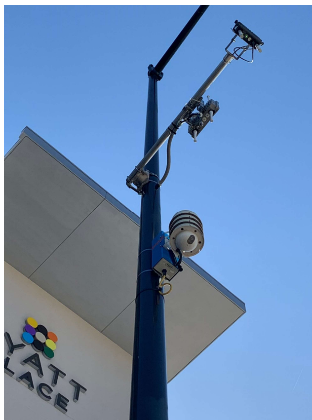
Figure 25 – Smart sensors at Peña Station
