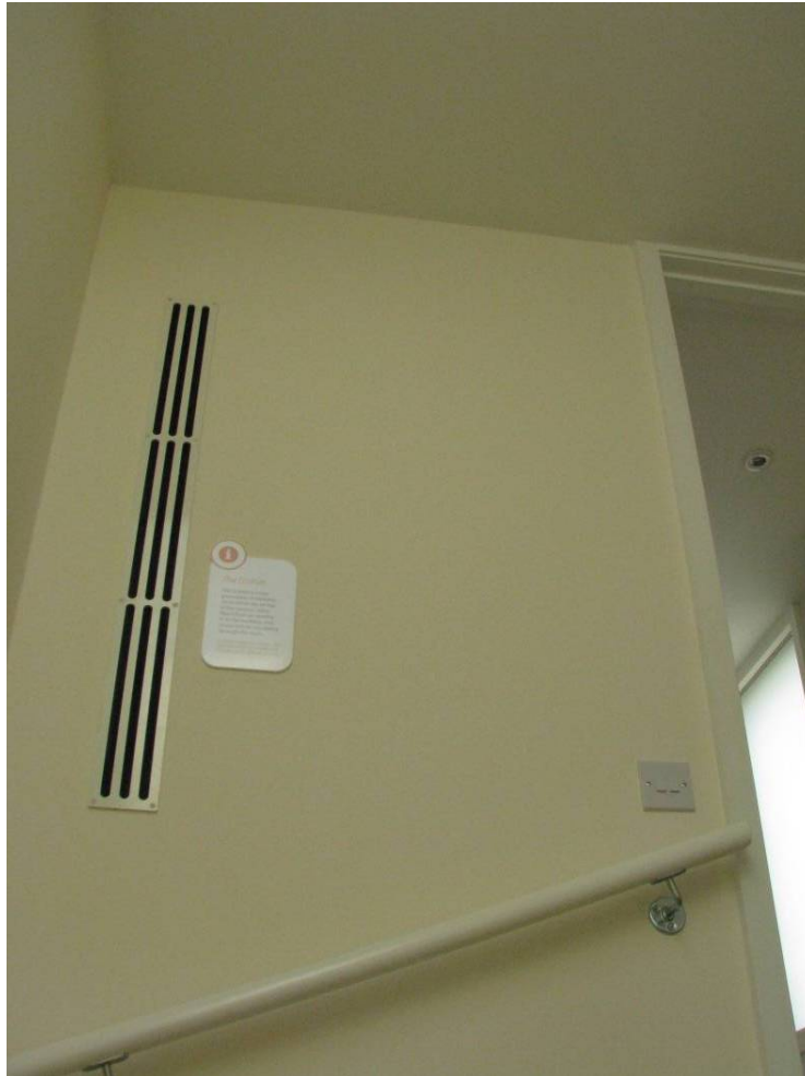
Oxley Wood, Milton Kenes, United Kingdom, September 2008 (Exhaust flue for Eco Hat)
