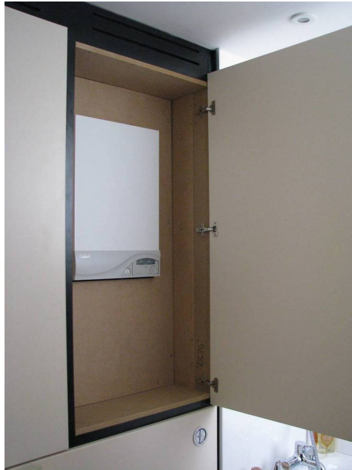
Oxley Wood, Milton Kenes, United Kingdom, September 2008 (Hot Water System)
