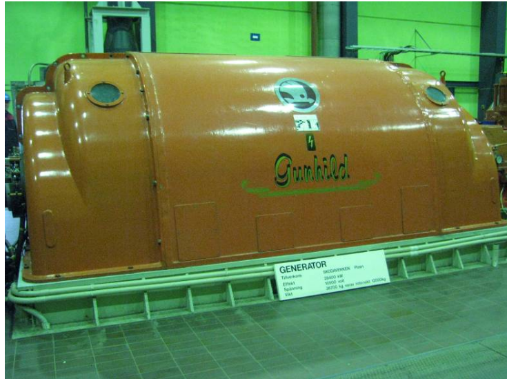
Vaxjo, Sweden, August 2008 (Generator – CHP Plant)
