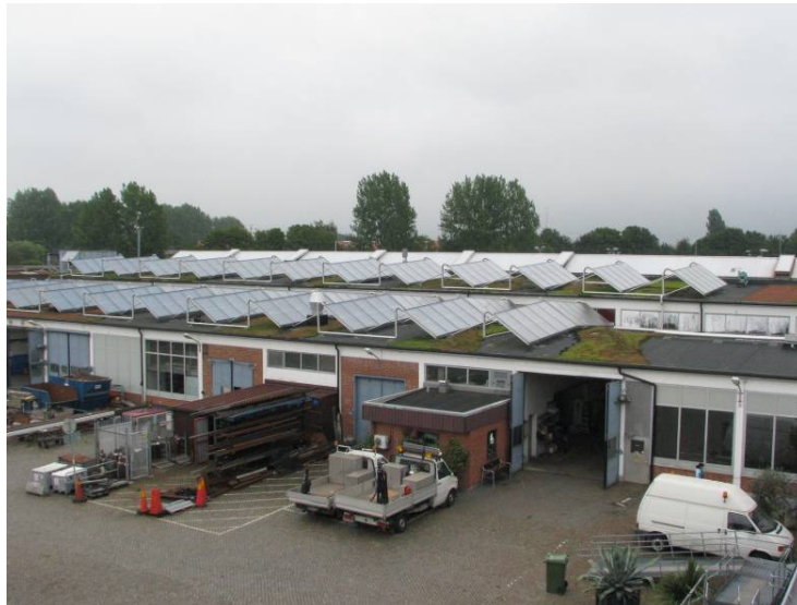
Solar hot water, Augustenborgs, Sweden, August 2008
