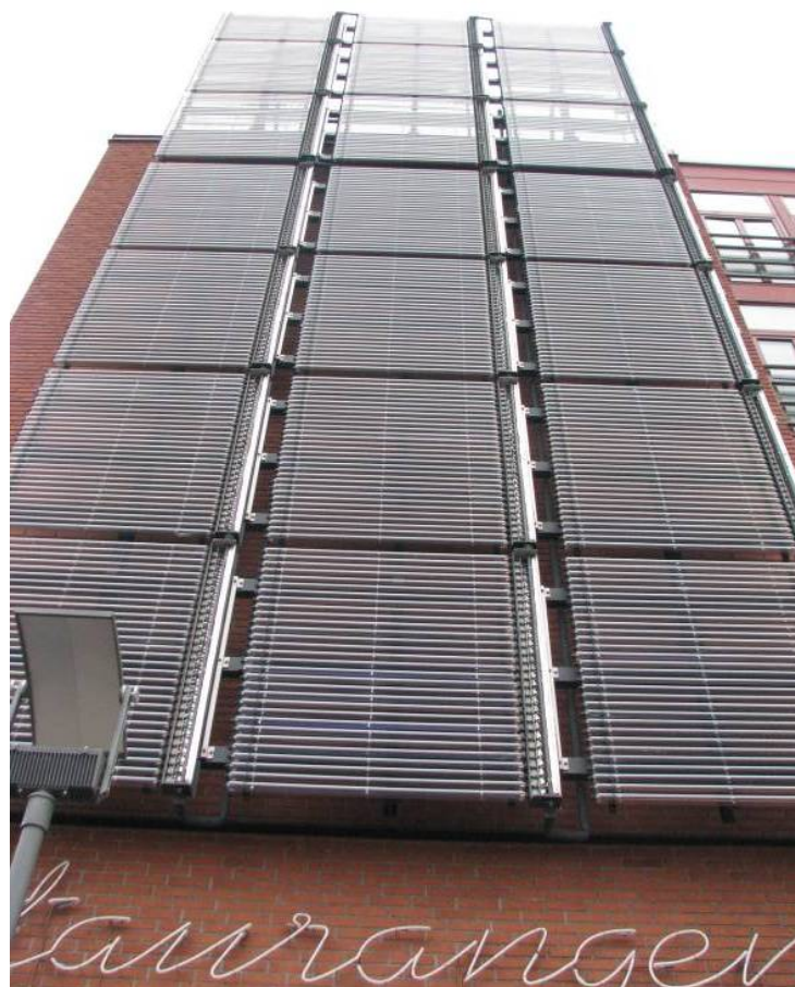
Evacuated Tube Solar Thermal Collectors, Malmo, Sweden, August 2008
