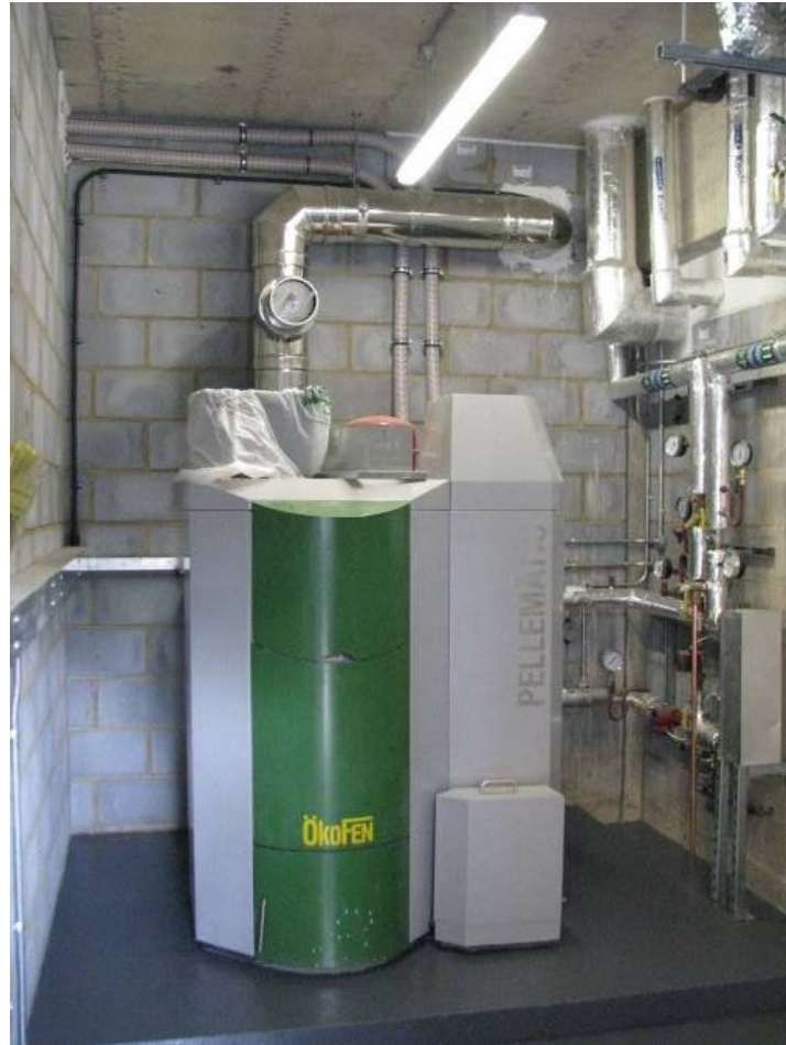
Greenwich Millenium Village, London, United Kingdom, September 2008 (Biomass Boiler)
