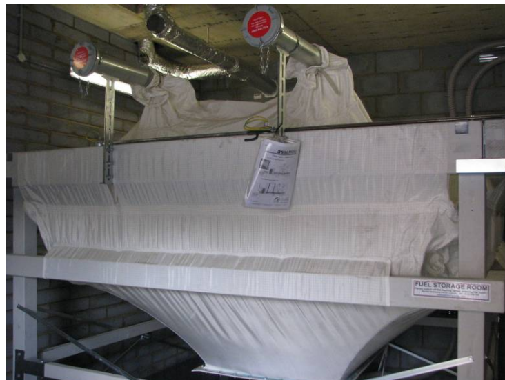
Greenwich Millenium Village, London, United Kingdom, September 2008 (Wood pellet biomass hopper)
