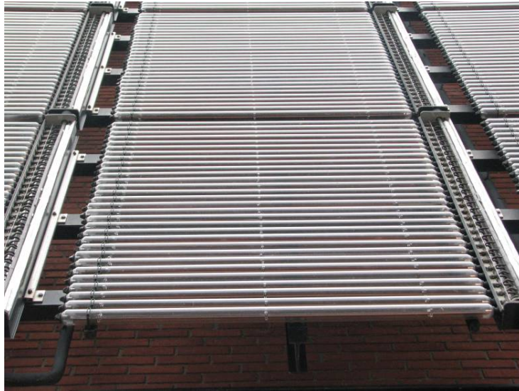
Evacuated Tube Solar Thermal Collectors, Malmo, Sweden, August 2008
