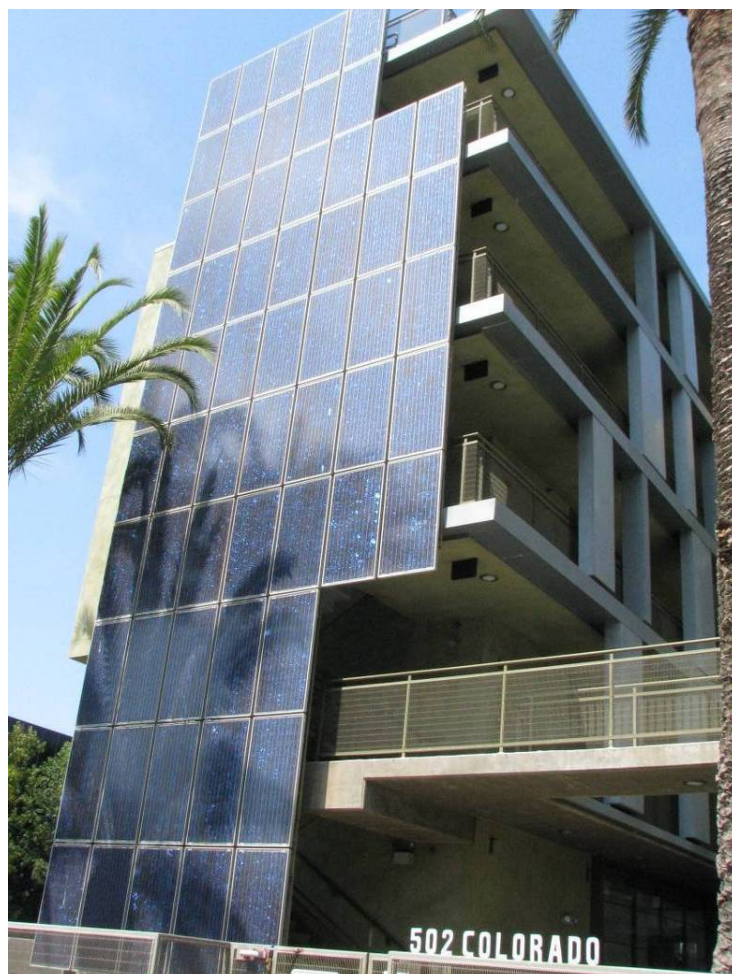
Solar Panels, 502 Colorado Road Santa Monica (Affordable Housing), United States of America, August 2008
