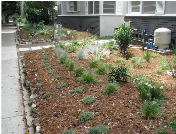
Stormwater Irrigation System, Santa Monica, United States of America, August 2008
