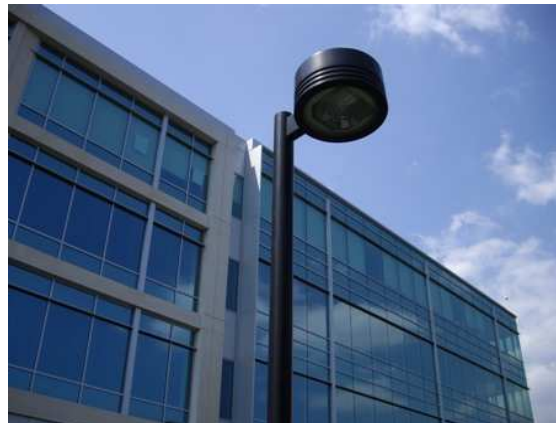
Photo 12 - LED - Street Lighting
