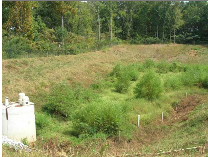
Detention Pond – City of Griffin - showing risers for flushing of the Agricultural drains
