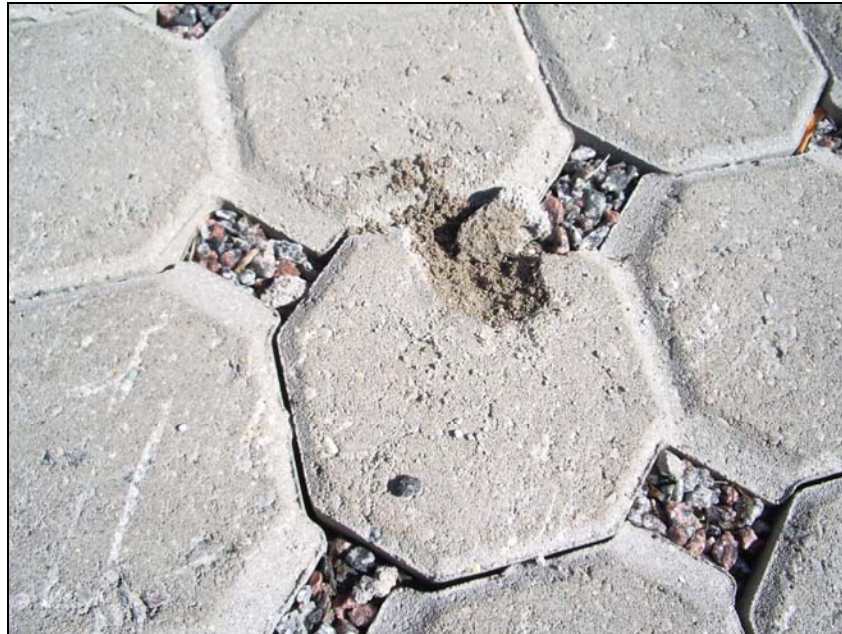
Close up view of the permeable pavement
