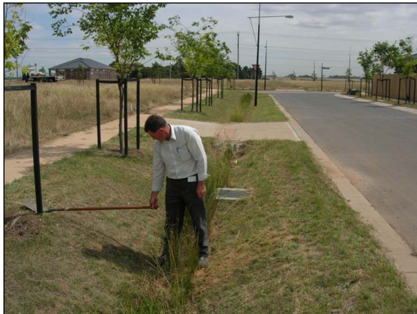
Bio-retention swale at Wyndham Waters Truganina – highlighting non - maintainable batters.
