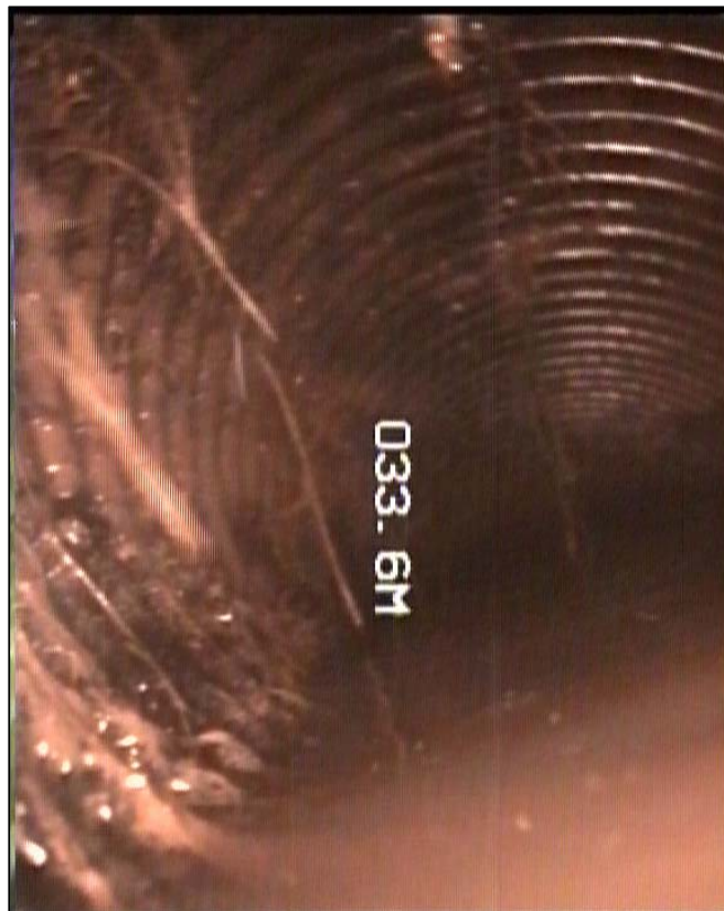
Roots shown entering the 100mm dia. Agricultural Pipe in the Bio-retention System within 12 months of construction
