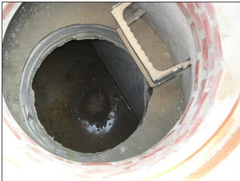
Below ground sand filter- Baltimore County
