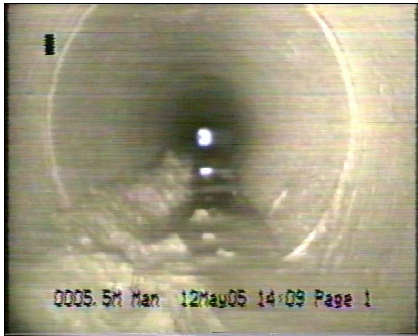
Sediment in a 300 mm dia. pipe after the pipe had been flushed on completion of the construction of the subdivision.
