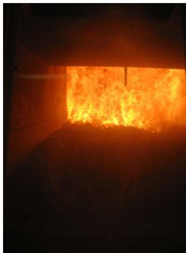
Photo IMG-0110 Incineration Chamber
