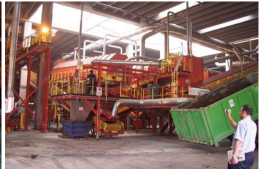
Plant and Conveyor System
