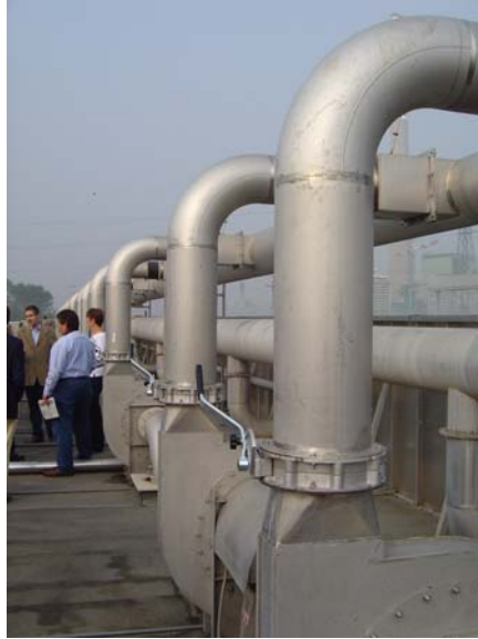
Air Extraction Units
